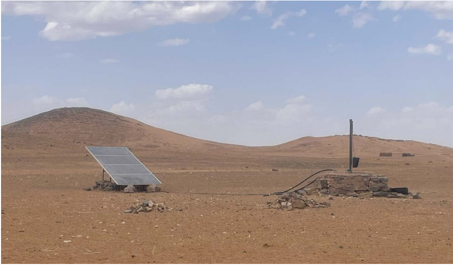
A motorized pump that uses solar power to generate electricity. With more people opting for solar panels, such pumps can be found across Morocco.
